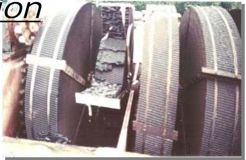
Collapsed Rotor Assembly
