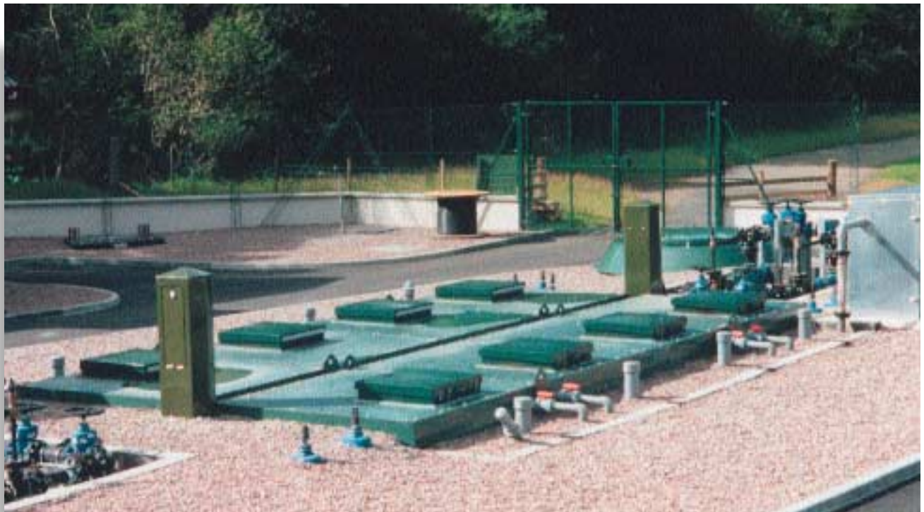
Below ground wastewater treatment works, population equivalent 1500.
