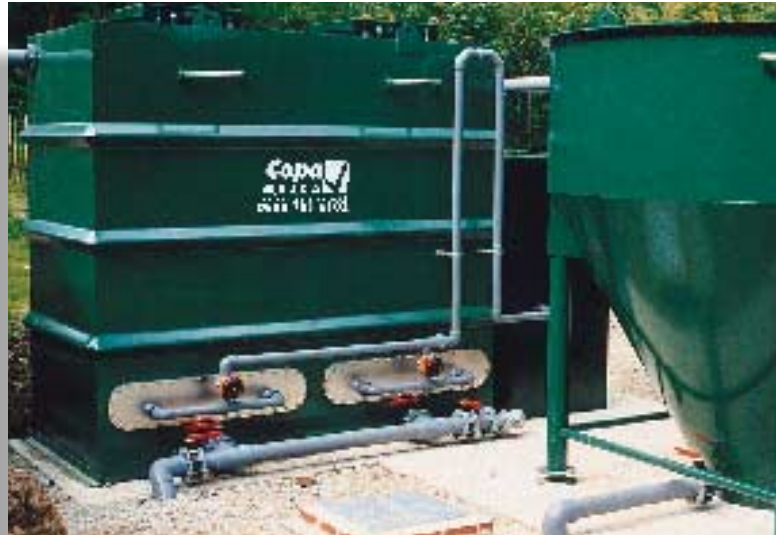
Above ground wastewater treatment works, population equivalent 150.
