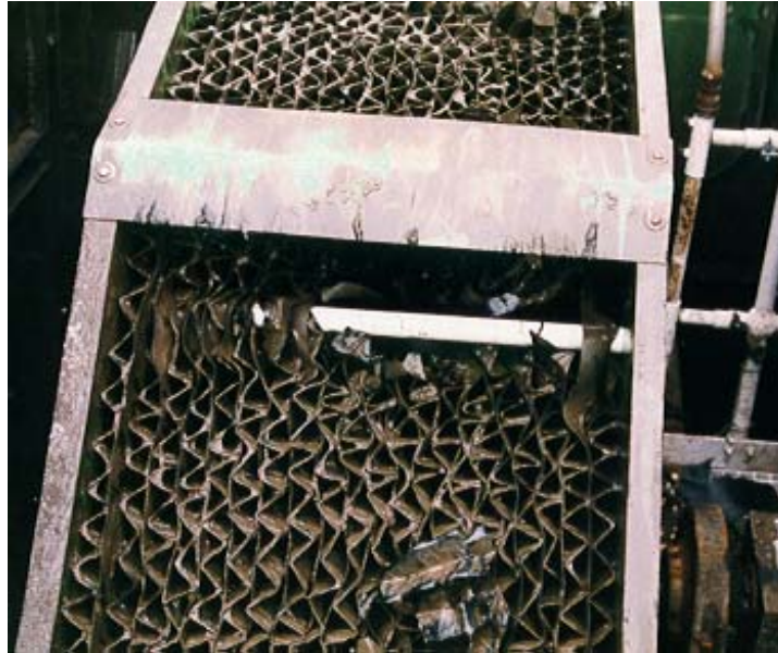
Figure 6 Loss of media pack due to tearing of HD polypropylene media panels
