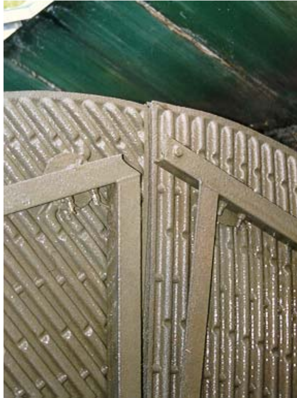
Figure 2 Damaged media support structure
