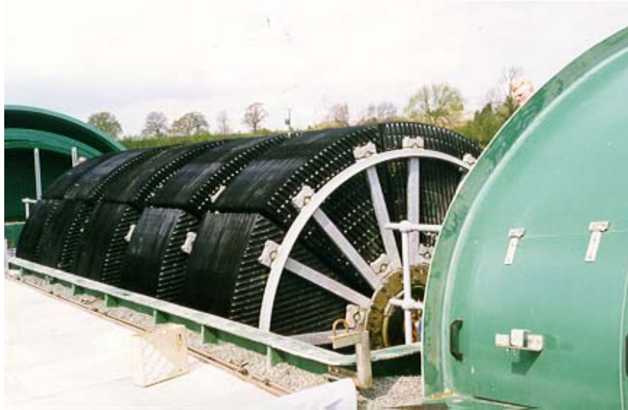
Figure 1 Typical Rotating Biological Contactor
