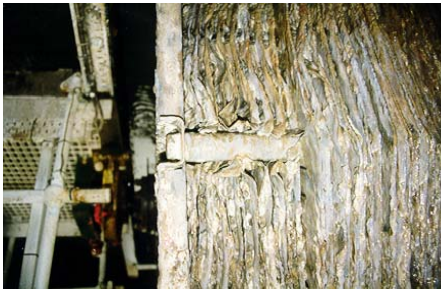
Figure 5 Tearing of high-density polypropylene media panels
